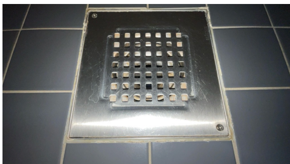
Sluk under slukrist.
