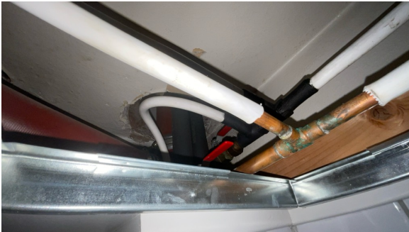
Kobberrør. To stoppekraner.
