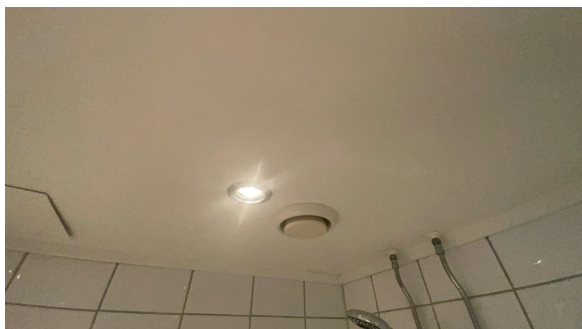
Lufteventil i himling.
