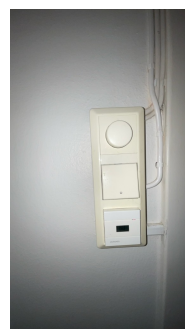
Termostatbryter for varmekabler.
