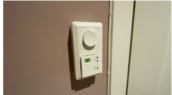
Termostatbryter for varmekabler.
