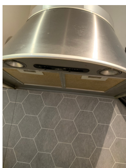
Kullfilterventilator over kokesone
