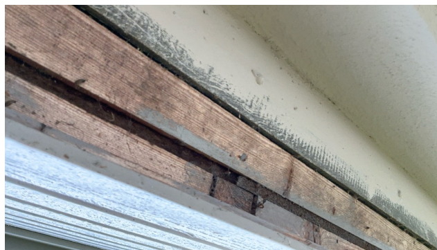
Det mangler lufting underside panel
