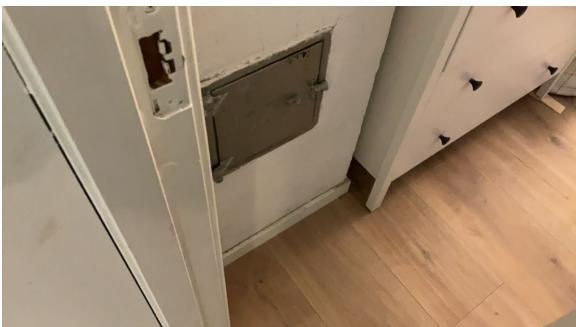
Manglende Ildfast plate under feieluke.
