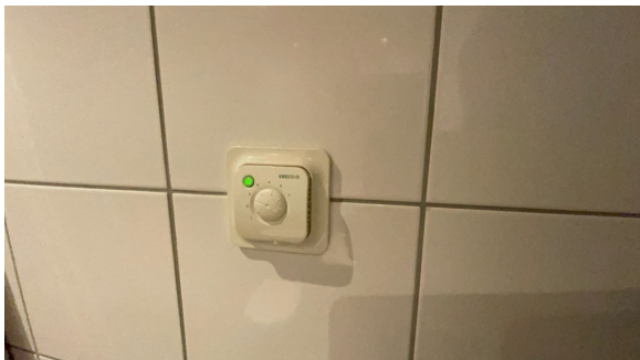
Termostatbryter for varmekabler.
