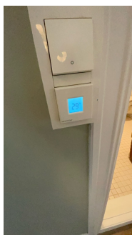
Termostatbryter for varmekabler.
