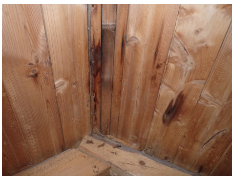
Skjolder i undertak
