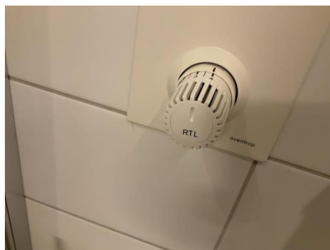
Regulator gulvvarme bad
