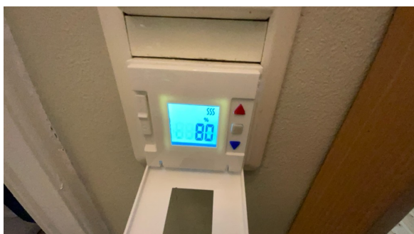
Termostatbryter for varmekabler.
