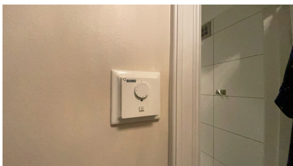
Termostatbryter for varmekabler.
