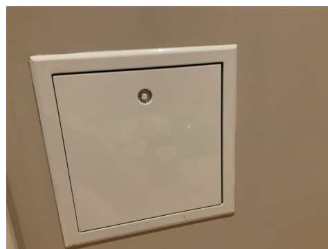
Regulator gulvvarme bad bak luke
