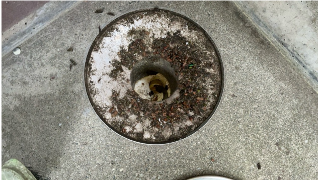
Sluk for avrenning overvann
