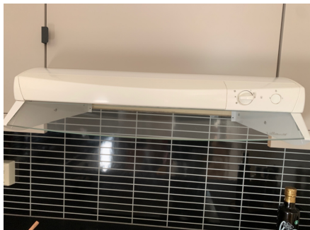
Spjellventilator over kokesone
