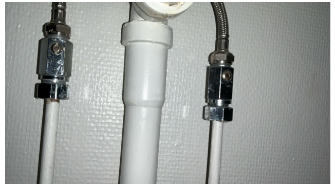
Stoppekraner servant bad
